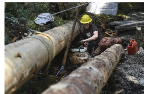
Duncan Campbell, of Trail Mix, works on a log bridge for a new Treadwell Gorge reroute trail on the Treadwell Ditch Trail. Source: Michael Penn | Juneau Empire
