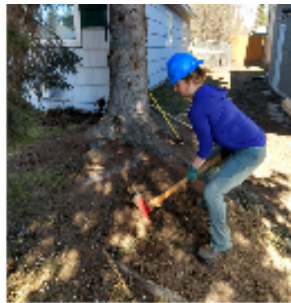
GRUBBING -Grubbing is decompacting material in the ground using the adze end of a pulask or another grubbing tool -Bend at the knees and keep a straight spine -Stop work if you notice pain, numbness, or tingling in hands
